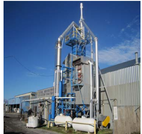
Pilot Plant & Baghouse
