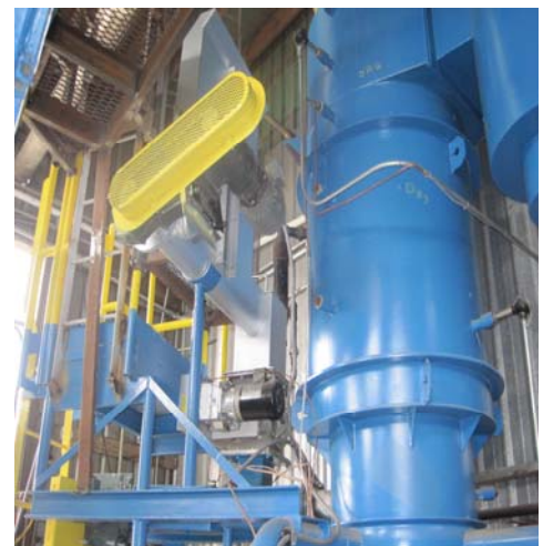
New Pyrolysis Unit
