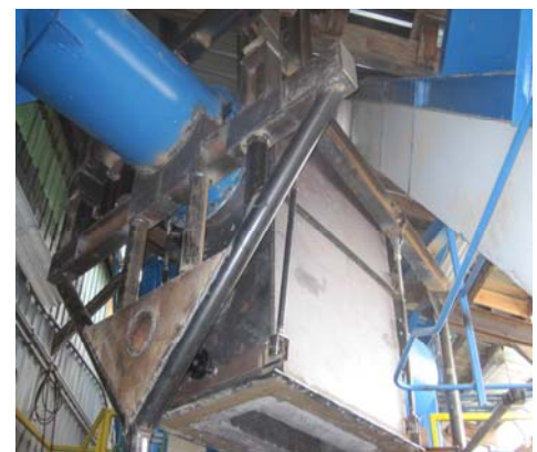
Gas Cooler / Boiler
